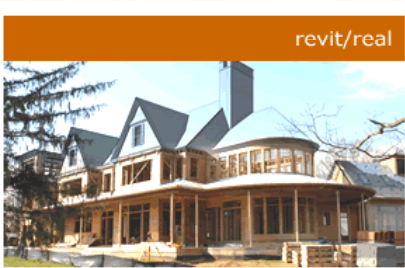
Overlay of Revit Model and Real-World Construction Waterfront Residence in Annapolis, MD
